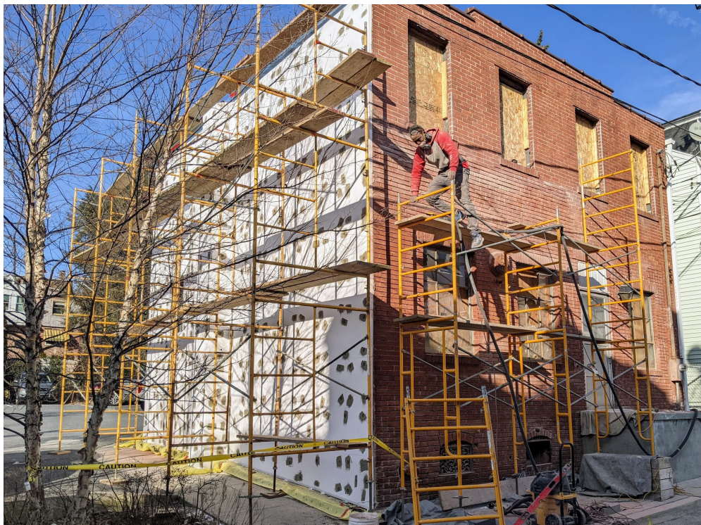
Repointing brick on front, installing stucco cladding system on side of building (EIFS-External Insulation and Finishing System. The first layer is foam board followed by a fiberglass mesh and a finishing coat.
